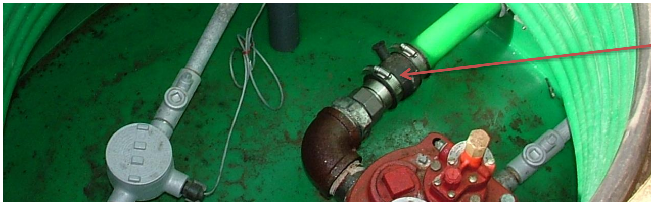
Test boot located in a sump
