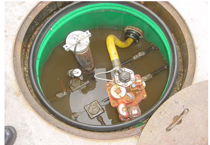
Contained turbine sump full of liquid
