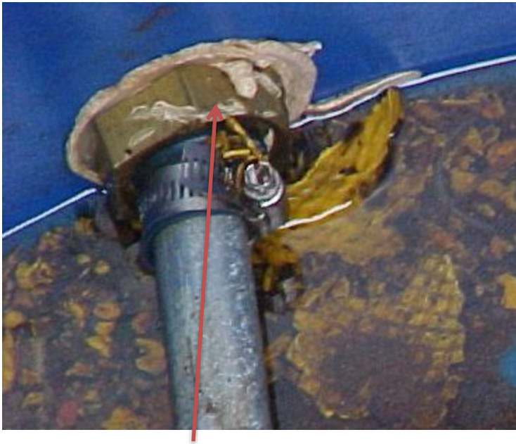
Sump penetration seals in poor condition
