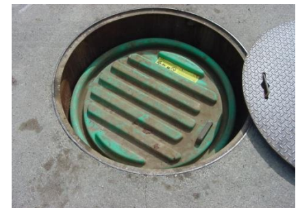
Circular steel sump lid pulled back to show the inner lid covering the turbine sump
