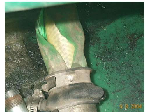
Flexible piping is cracked
