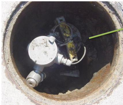
Uncontained Equipment Sump
