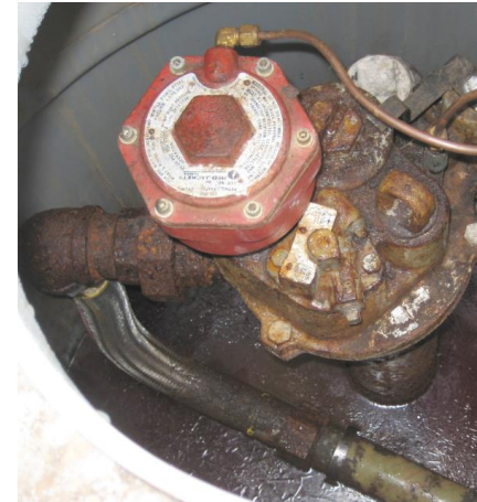
Corroded metal piping
