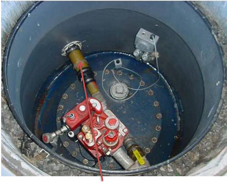
Tank top sump showing fiberglass piping.
