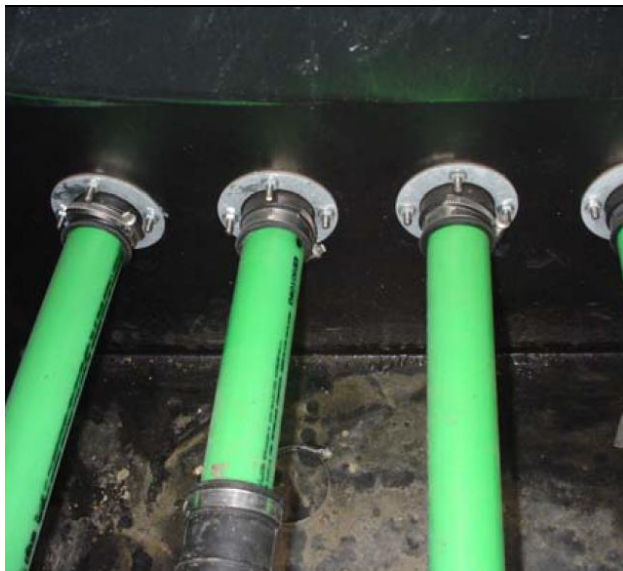
Flexible plastic piping
