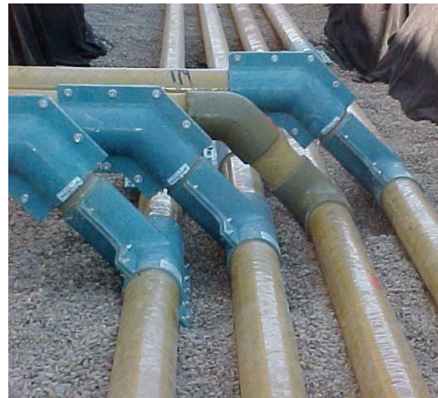
Non-flexible fiberglass reinforced plastic piping
