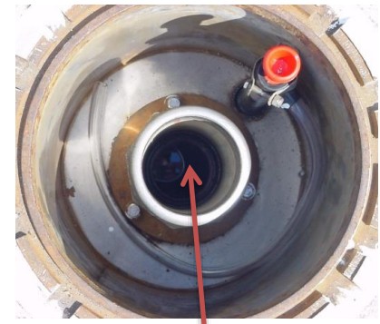
Drop-tube shutoff valve can be seen in the fill pipe
